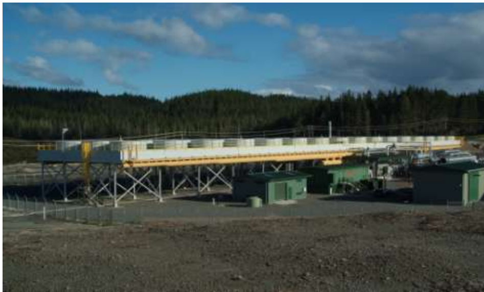
Figure: Station 2, 15 MWe Ormat binary plant commissioned in 2008
