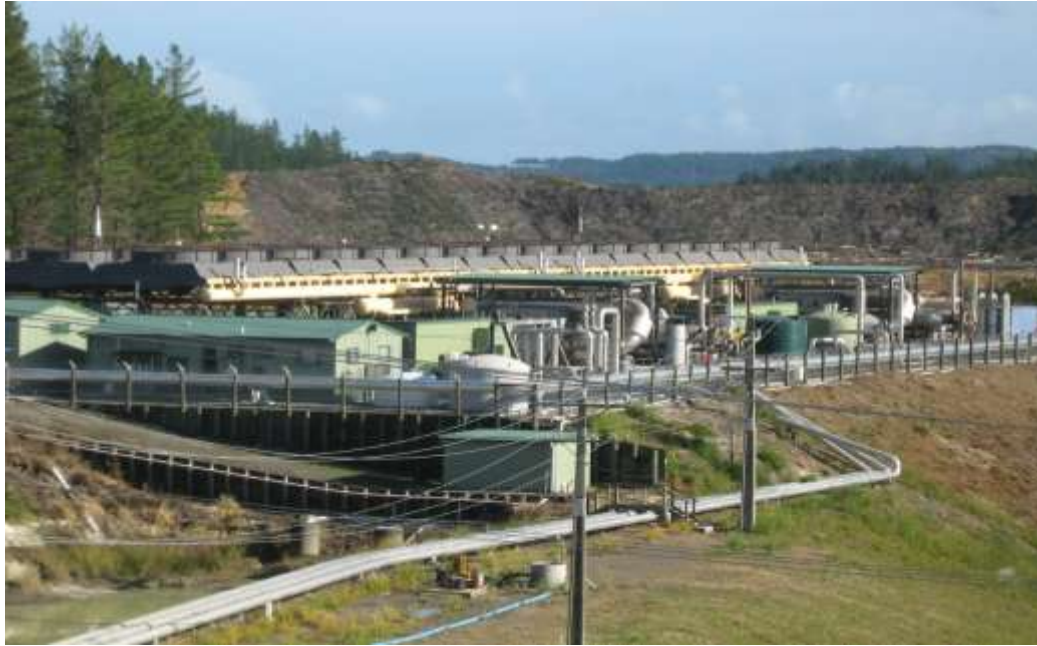
Figure: Station 1, 10MWe Ormat binary plant commissioned in 1998
