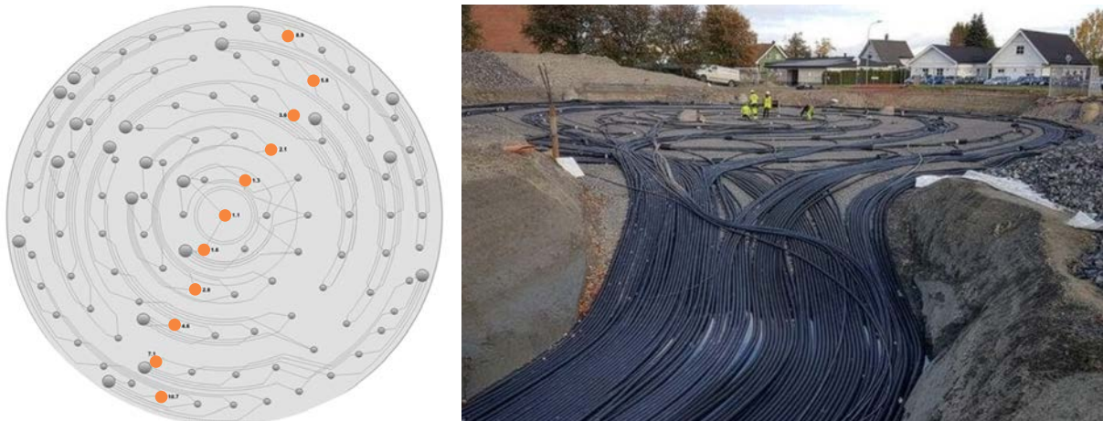
Figure 10 Top of the BTES. 11 fiber optic string locations shown on the LHS diagram in the small orange circles. RHS supply and return piping from the bore holes in the BTES covered over with the car park on top when it was completed.
