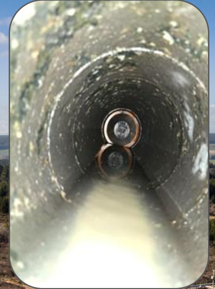
Pipe line downstream of Northern Plant
